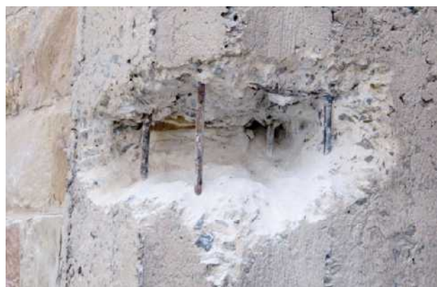
Figure 6: Damage caused to connect all reinforcement, including those located in non-carbonated areas
