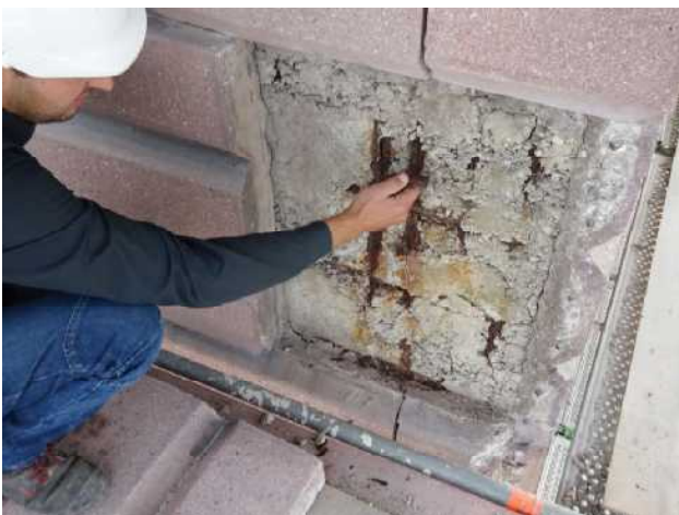
Fig. 3: See 3.1.2: Honeycombs and larger voids in the back of the lost in architectural concrete
