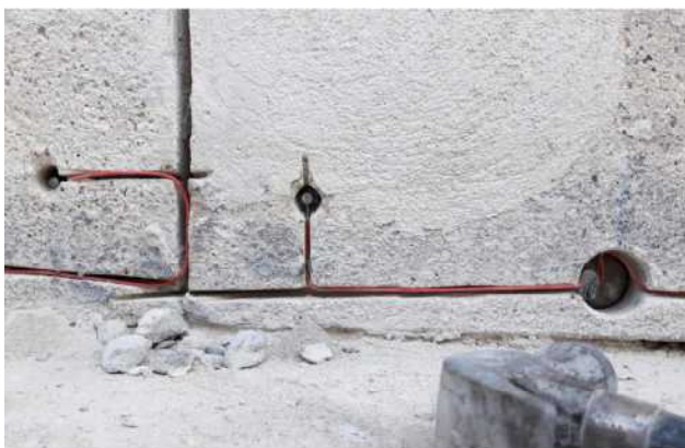
Fig. 7: To limit the damage by finer techniques of search and connection of reinforcement, limited to those located in the carbonated or potentially carbonated concrete.
