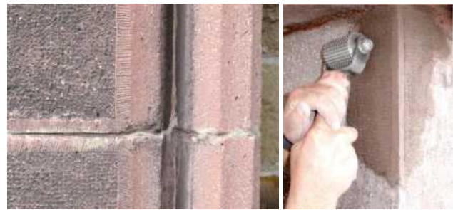
Fig. 9 and 10: On the left, the relief and the original stain on Art Deco architectonic concrete (1927). On the right, restoration of the relief in a fresh local repair with tools developed ad hoc.
