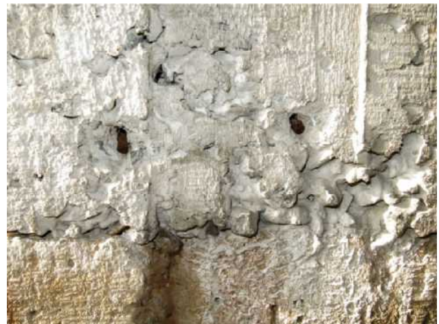
Fig. 4: Honeycombs above the retrieval joint; homogeneous but sparse concrete below the joint. The black dots in the gravel nest are rebars bare for 60 years, without expansive rust, despite their exposure up front
