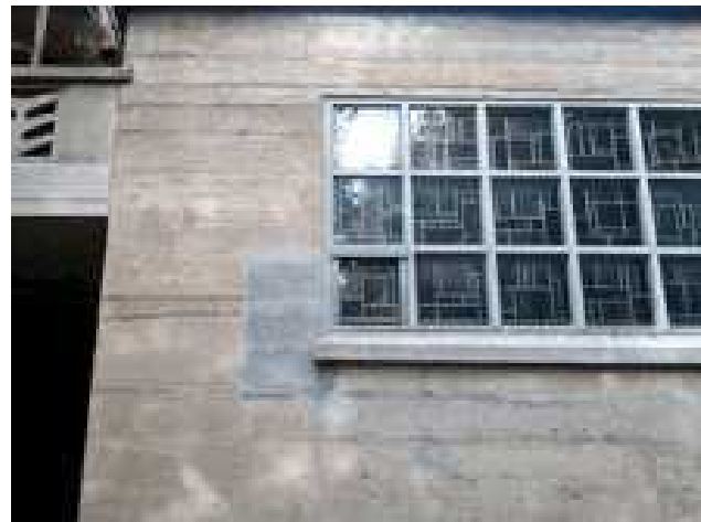
Fig. 2: The patch repair, made using modified mortar, ages differently (more blueish) than the original substrate.
